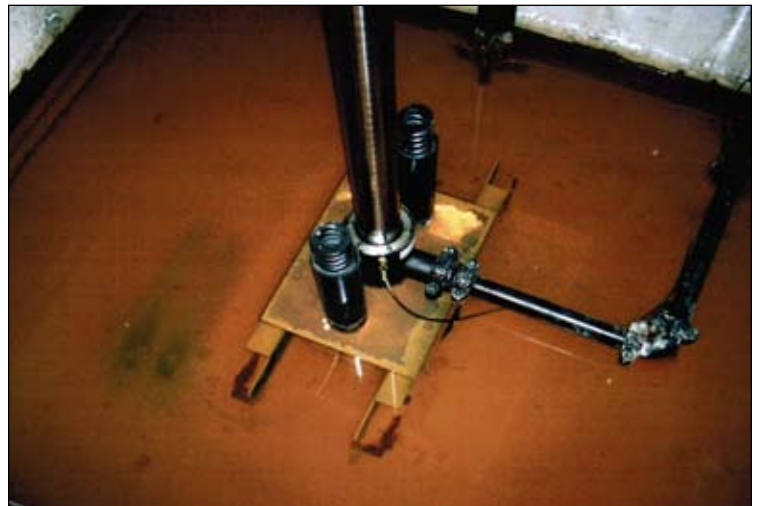
Elevator company had been unable to solve shaft flooding in campus building using their own personnel and resources.
