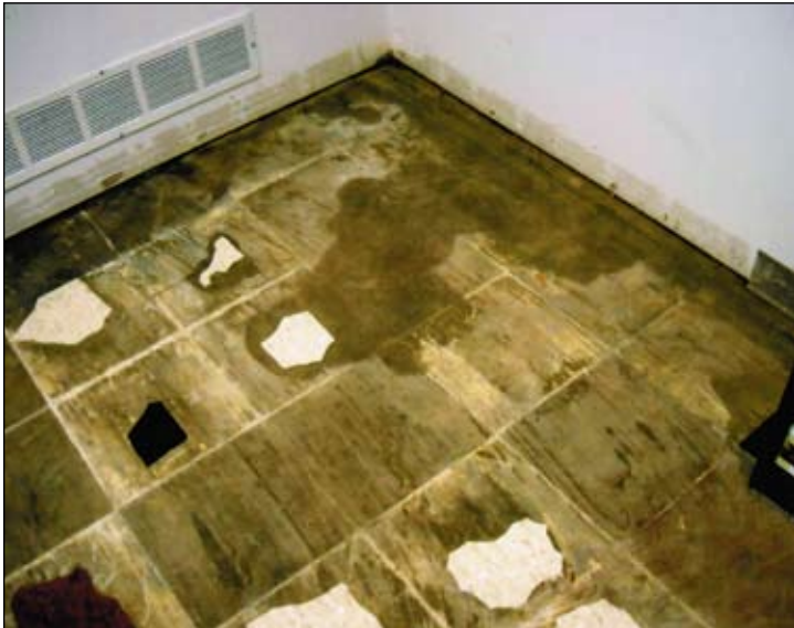
Basement infiltration affected the entire lower level of a college classroom building. A tissue dropped at the wall line would flow toward the center of the floor.
