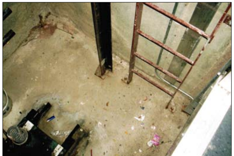
Curtain grouting contractor fixed shaft flooding within a day, and later also a similar problem in a mechanical room within a day.
