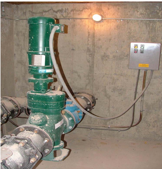
Each grinder, installed upstream of the concentrator in an 8 in. line, sees 400 gal/min of raw manure, for total of 0.5 mgd.
