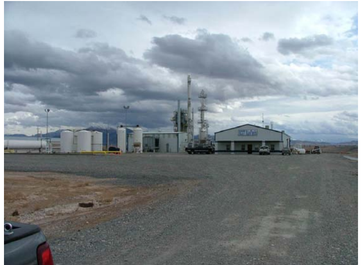
Installation of special grinder units eliminated recurrent pipeline blockages in new waste-to-energy plant.
