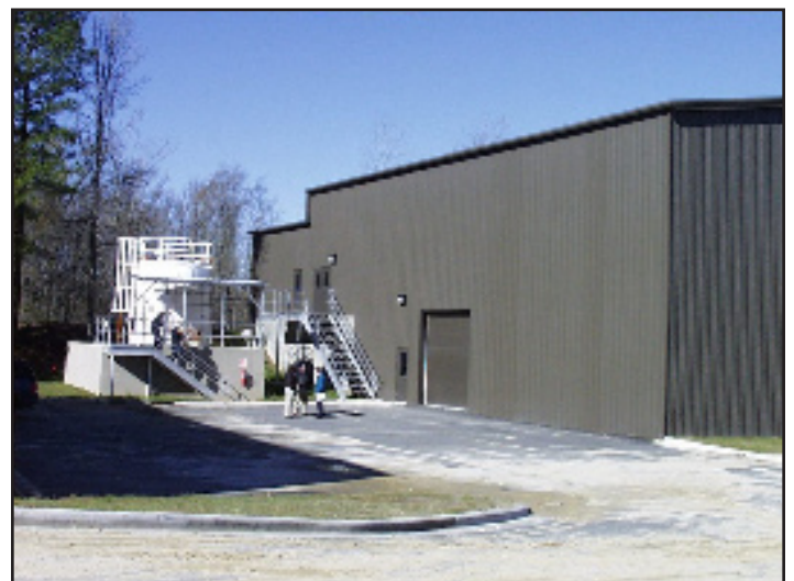
Filter operation includes addition of methanol to filter influent to provide organic substrate for a denitrifying microbiological culture in the filter media. Methanol is stored in an 8000-gal. tank.
