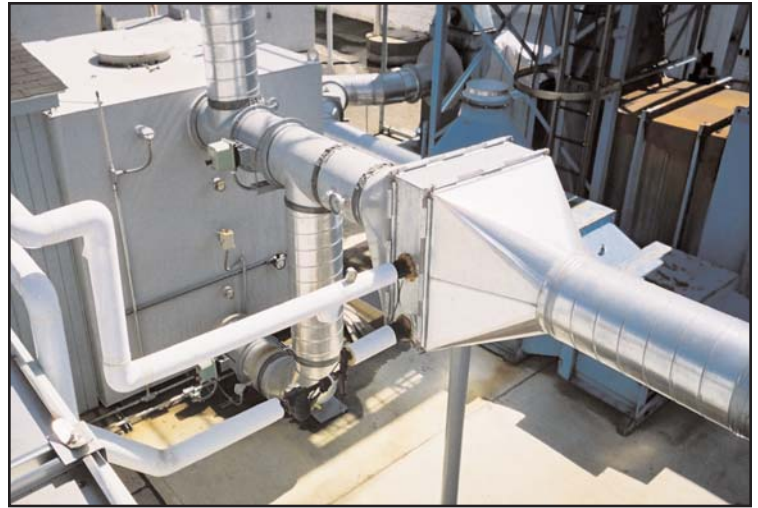
Actuators (green), controlling system dampers, were synchronized with actuators for dampers already in the plant. Heating coil in duct (square) provides for separation of VOC's from carbon, readying them for degradation in biofilter.
