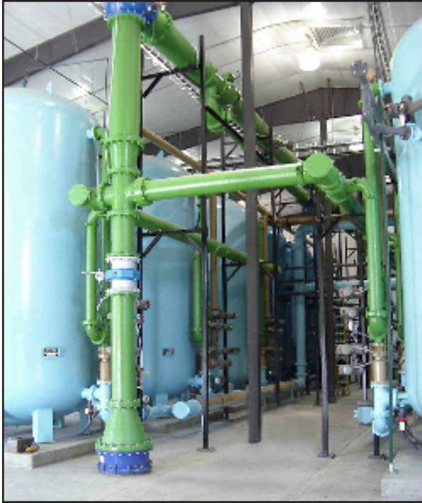
A computerized (PLC) control system operates 6 cation vessels and 6 anion vessels.
