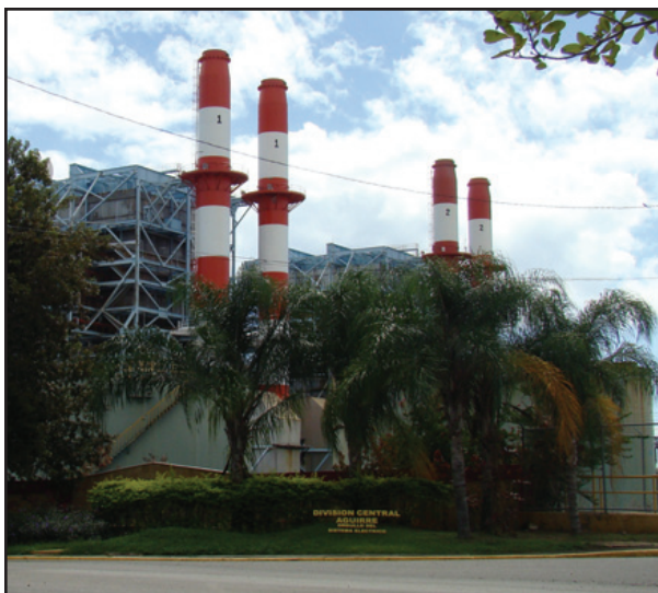
An IX DI system serves each of the plant's two 450 MW boilers. Each 1005 deg. F, 2600 psi boiler uses 1950 gal./min. of feed water, and requires 6000 gal./hr. of makeup water. Magnesium and calcium in the deep well feed water are now 420-450 parts per million (ppm), with chloride 80-90 ppm and silica 37 ppm.
