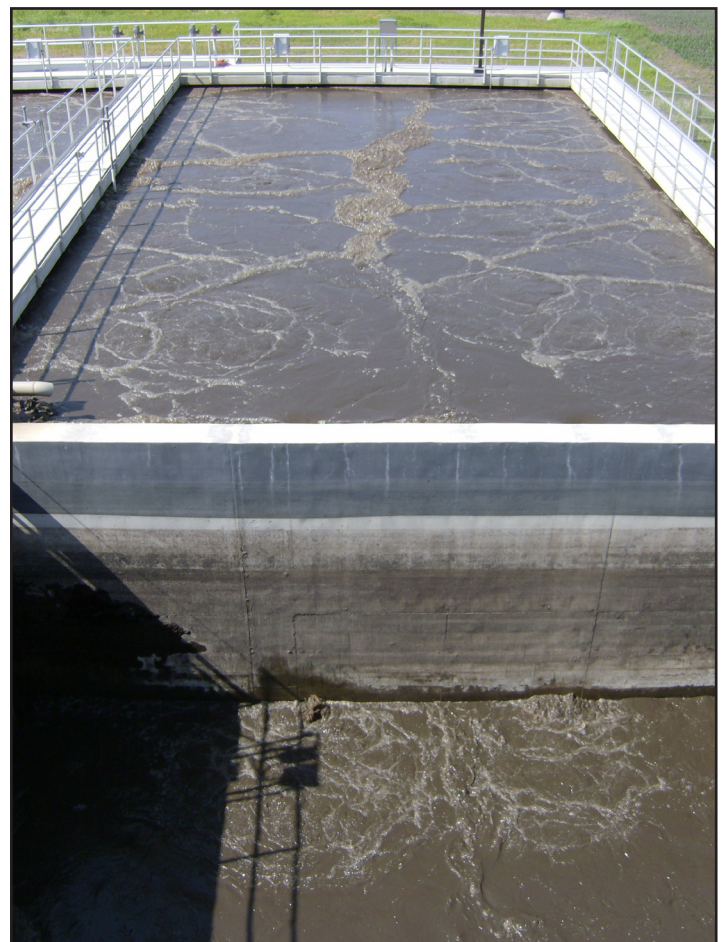
The surge/anoxic/mix (SAM ™ ) tank provides built-in flow equalization. It is preceded by a constant-level anaerobic selector chamber, and is followed by one or more SBR basins.
