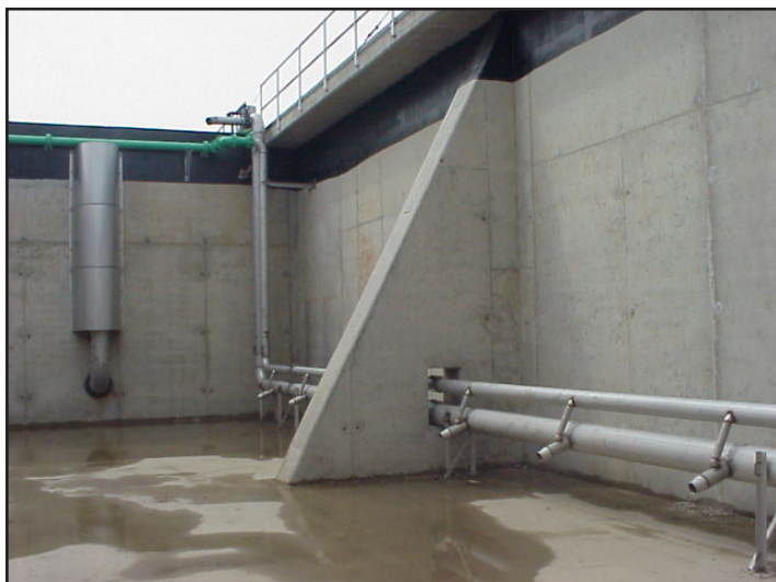
System includes in-basin jet aeration manifold and overflow weir/scum skimmer, shown here during installation.
